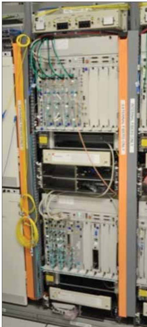
Figure 5. Photograph of the 100 Gb/s PM-QPSK prototype system in the field.
